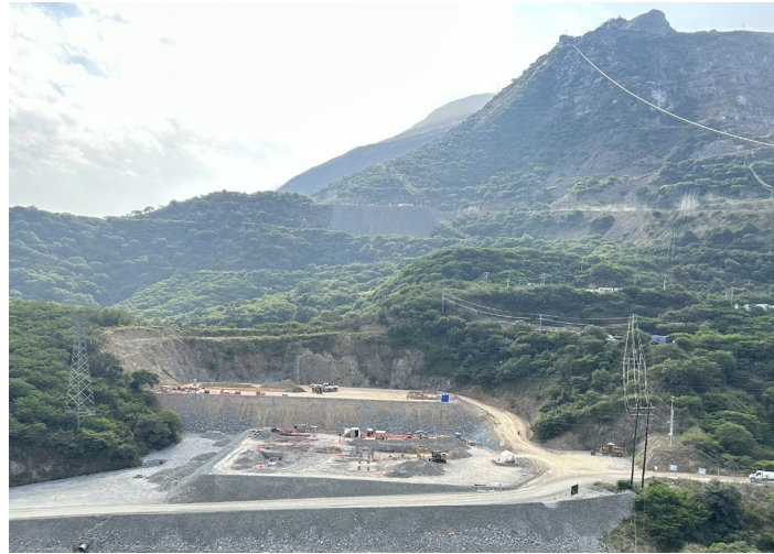
Water Treatment Plant and 230 kV substation
