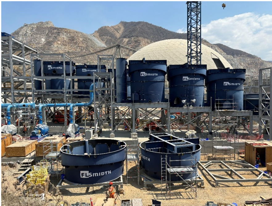
Figure 2: Construction of the flotation facility is progressing well with installation of the copper and iron sulphide flotation circuits and piping well underway
