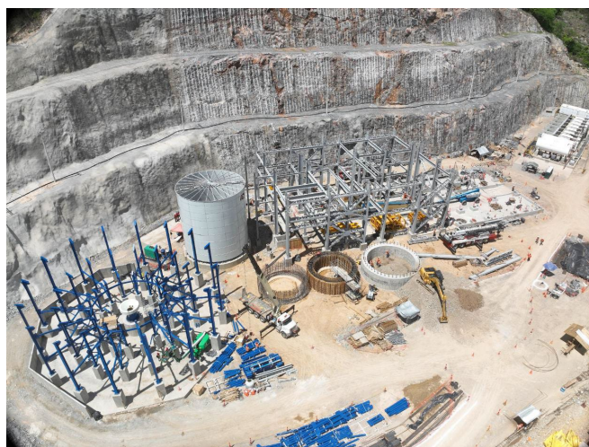
Figure 3: Construction activities at the paste plant, located outside of South Portal Upper
