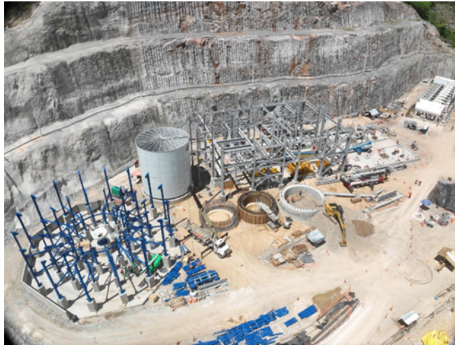
Figure 3: Construction activities at the paste plant, located outside of South Portal Upper
