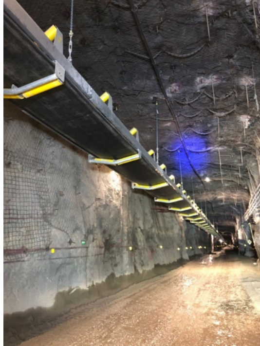
Figure 1: Installation of the Guajes conveyor belt has commenced following installation of conveyor tables
