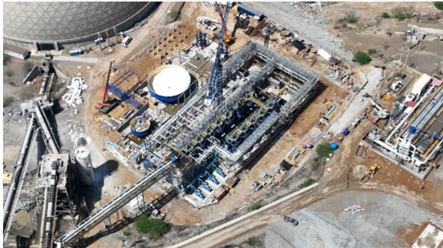
Figure 2: Construction activities at the flotation area, including the flotation tanks, thickeners, and regrind mills
