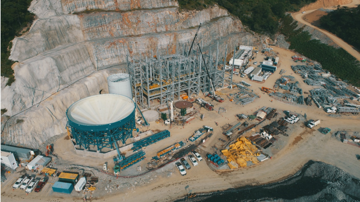
Figure 6: Construction of the binder silo, thickener, and building steel at the paste plant
