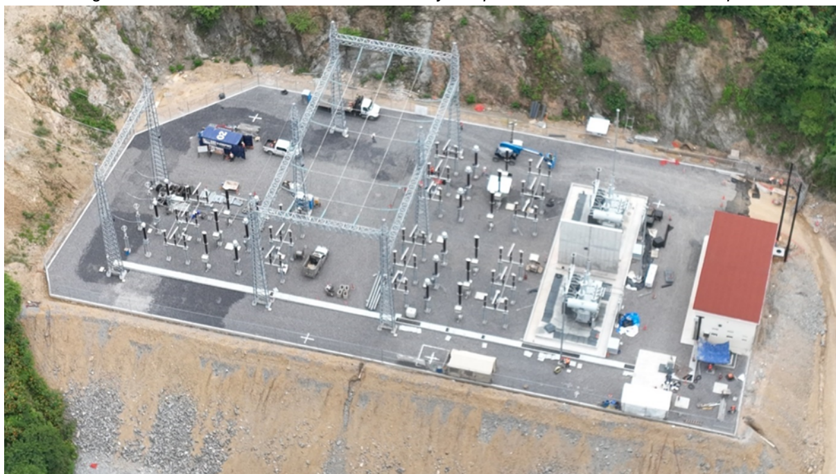
Figure 5: The 230 kV substation is substantially complete with main transformers in place
