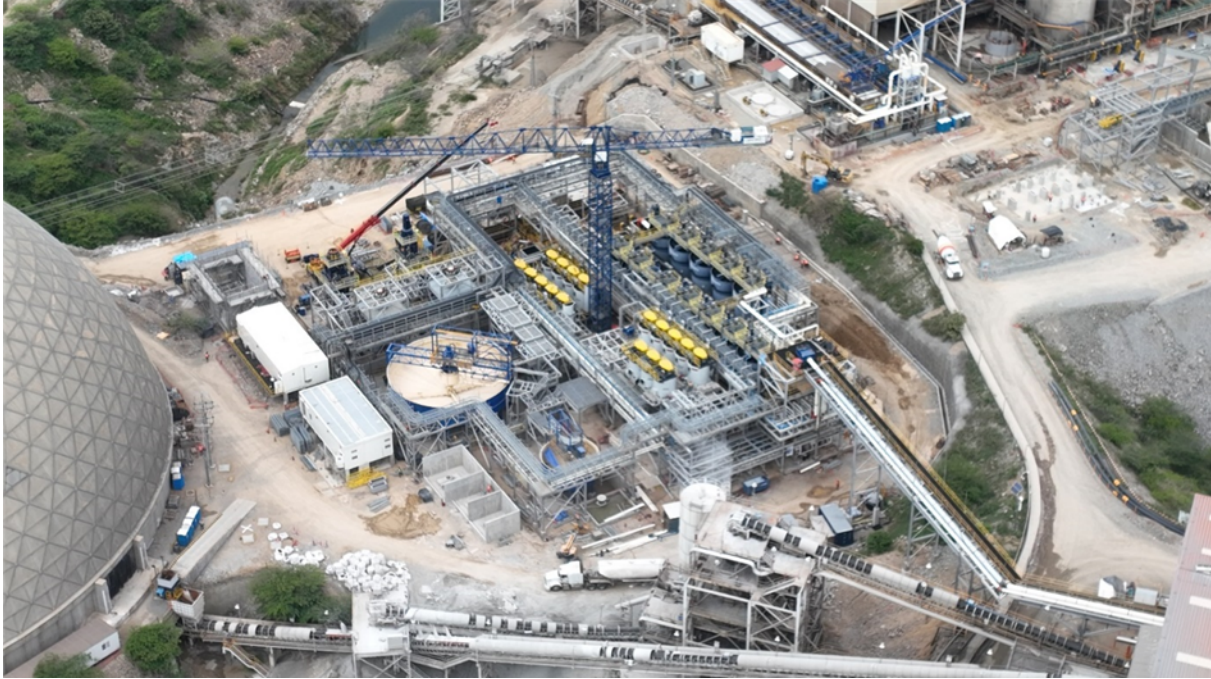
Figure 2: Construction of the flotation area is advancing, with both e-houses and associated cables now installed. Progress was also made on the installation of the regrind mill and cleaner cells.
