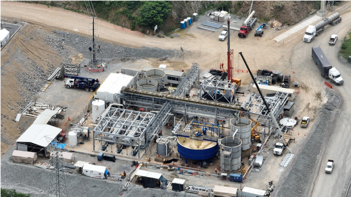
Figure 3: Construction of the water treatment plant is ongoing, with detox tanks for the first phase of water testing installed during the quarter
