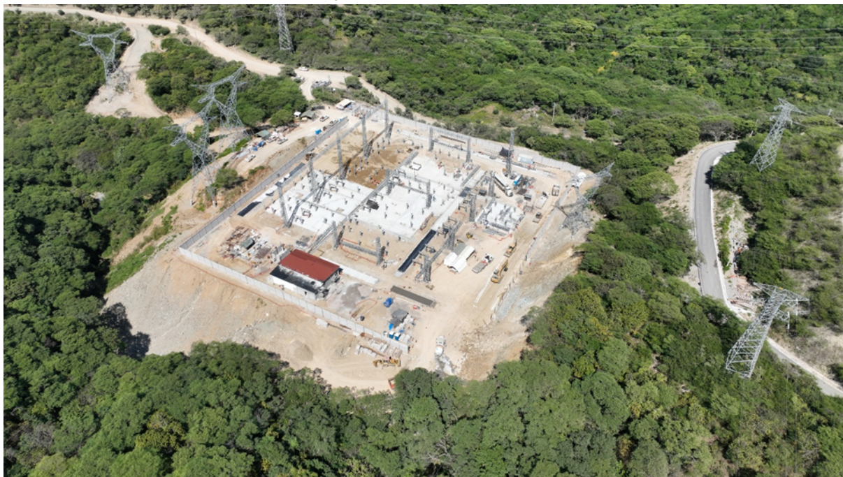
Figure 4: Galvanized towers have been installed at the 230 kV switchyard to support the transmission line between the yard and the substation
