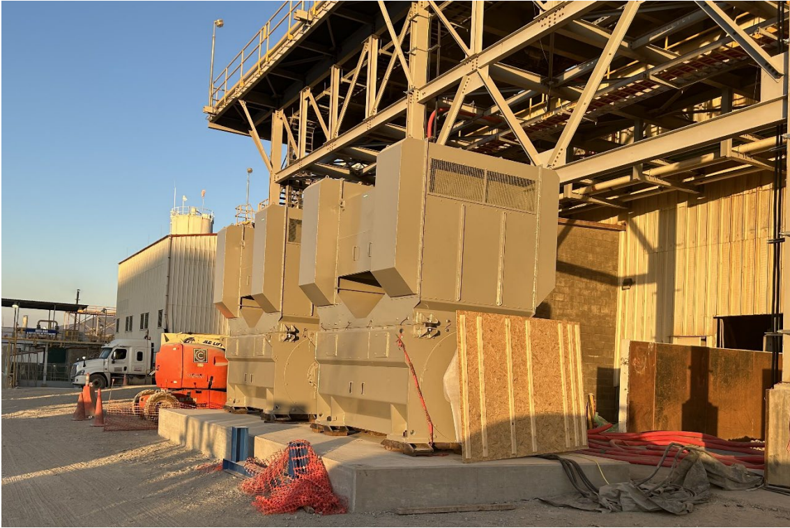
Figure 2: Pre-commissioning of the ball mill's variable frequency drives took place in December in order to mitigate potential risks during the tie-in period in February.
