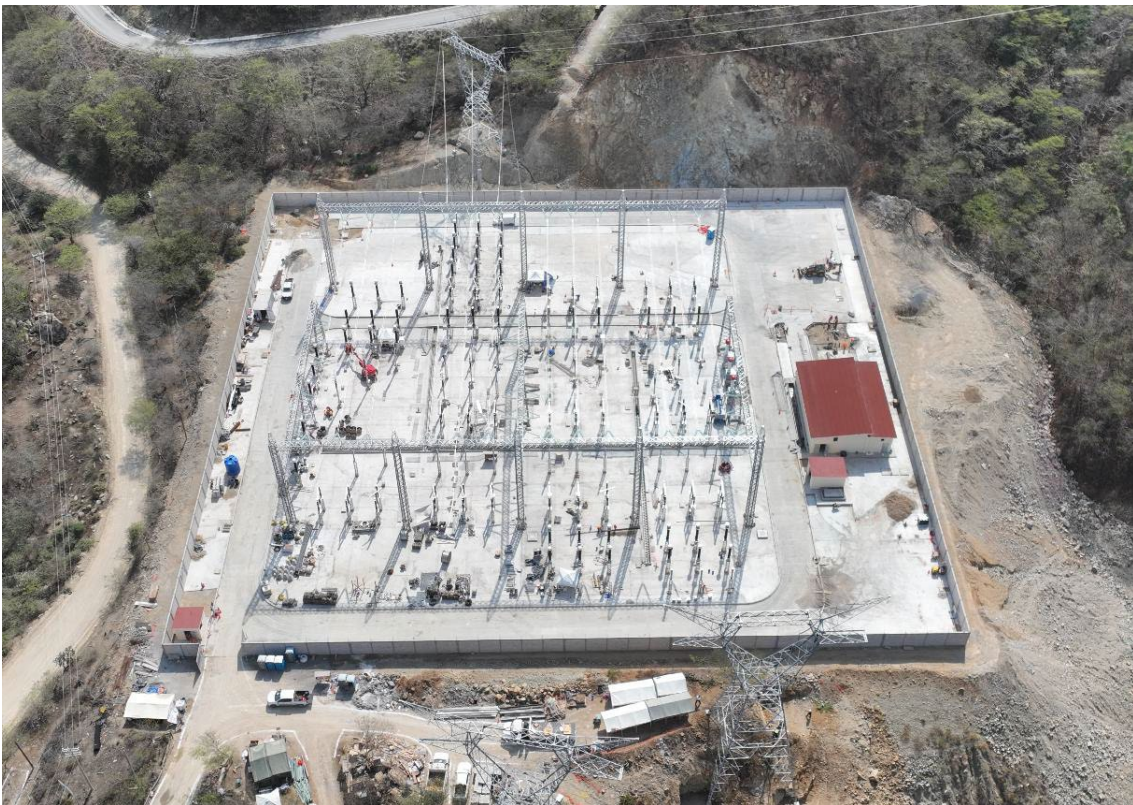
Figure 3: Transmission lines between the 230 kV switchyard (pictured below) and substation were connected in the quarter.
