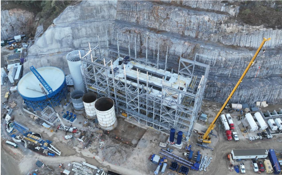
Figure 4: Work progressed on the paste plant during the quarter, including continued erection of the binder silo, thickener, and building steel.
