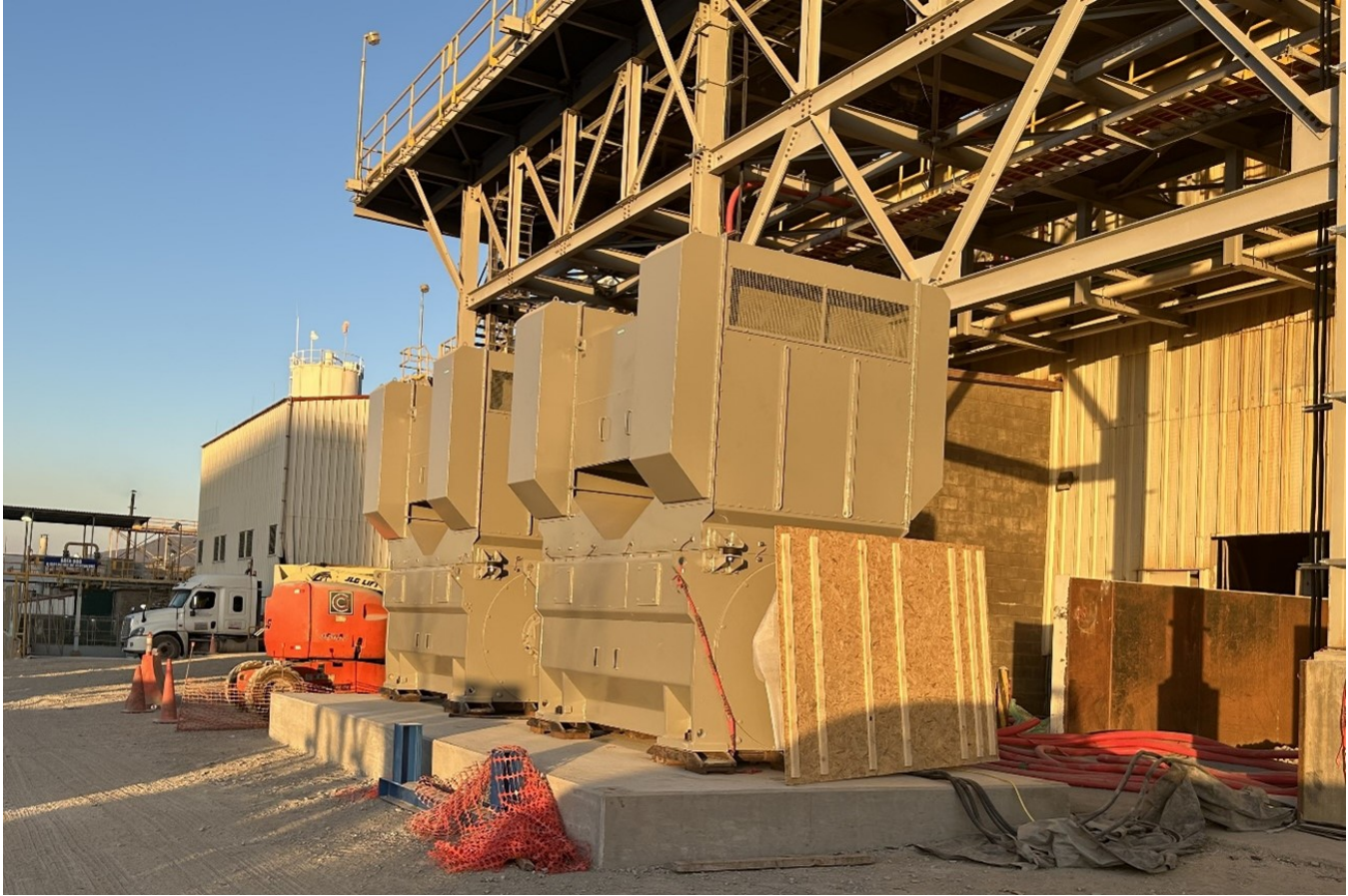
Figure 2: Pre-commissioning of the ball mill's variable frequency drives took place in December in order to mitigate potential risks during the tie-in period in February.
