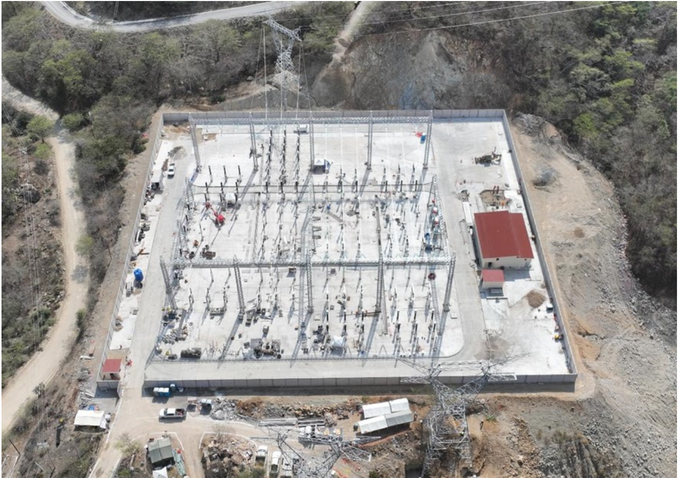
Figure 3: Transmission lines between the 230 kV switchyard (pictured below) and substation were connected in the quarter.
