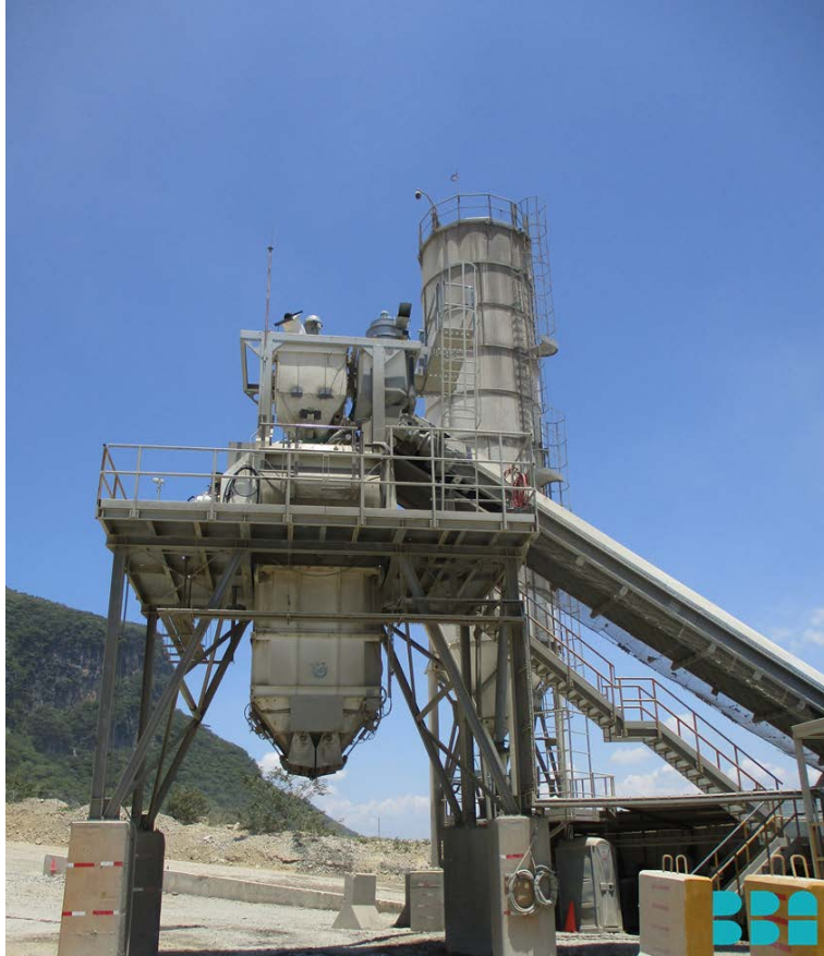
Figure 16-58: Backfill Mixer and Cement Silo
