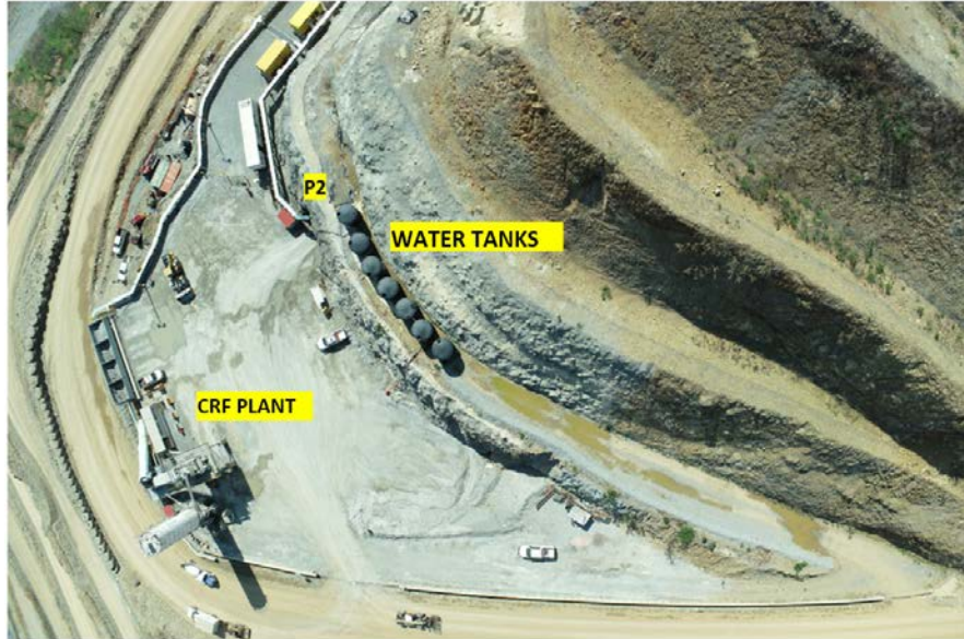
Figure 16-70: Portal 2 Water Tanks
