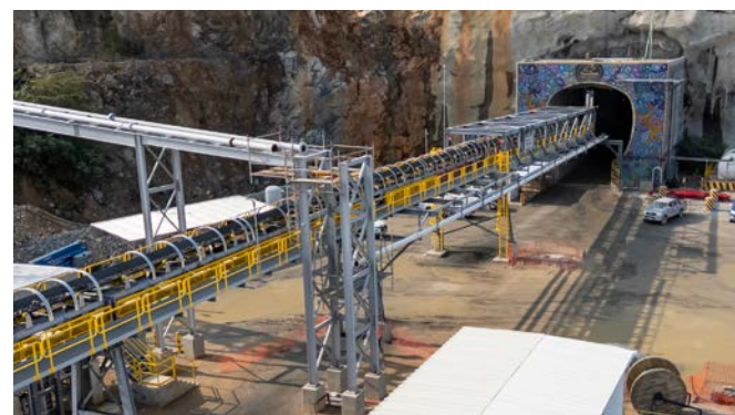
The Guajes Tunnel Conveyor
