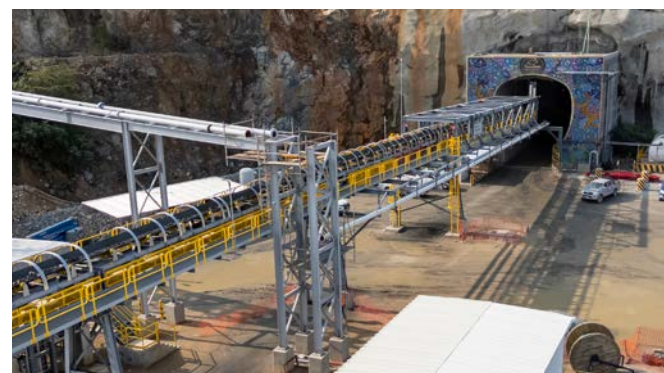
The Guajes Tunnel Conveyor
