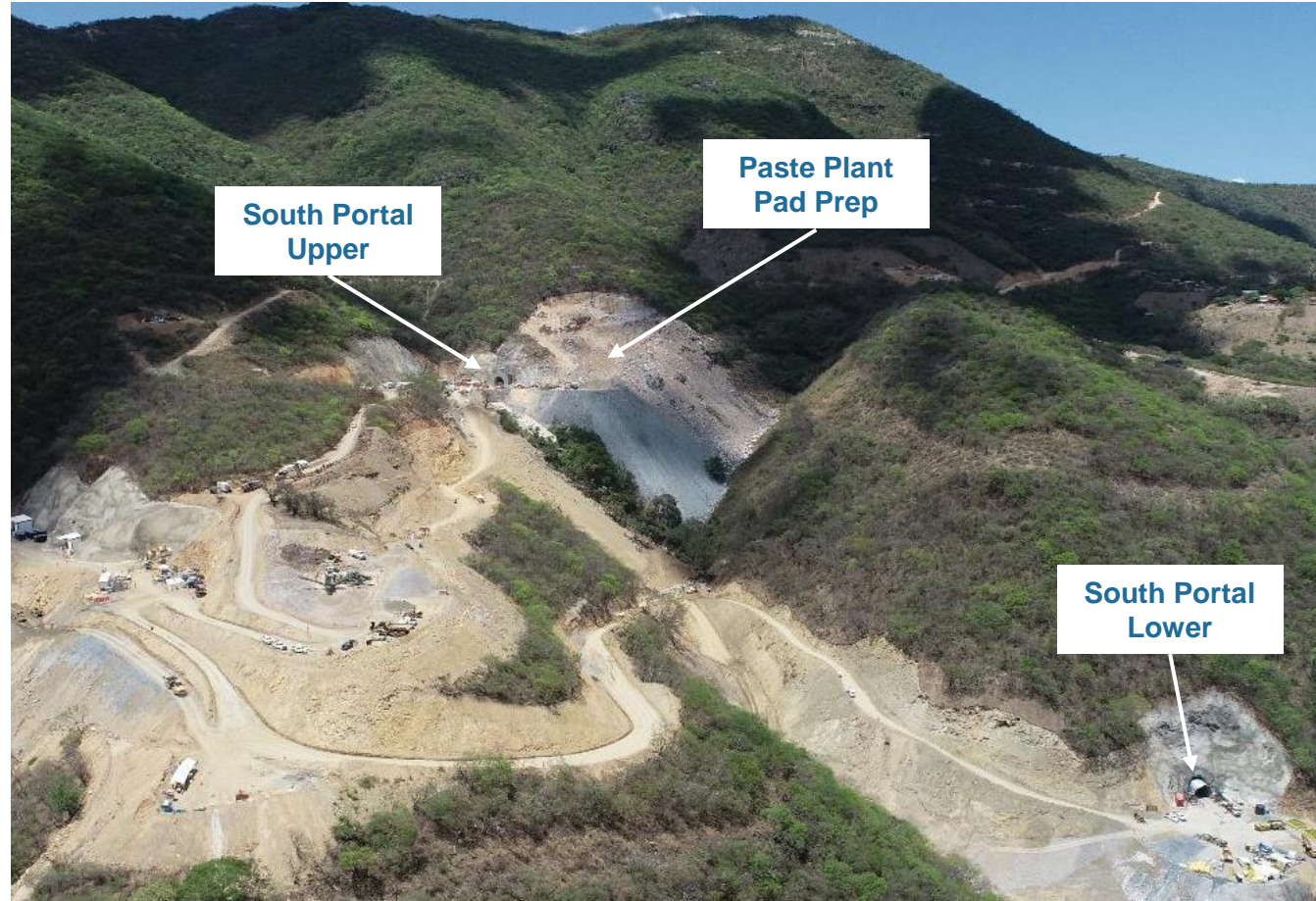
Earthworks on southside progressing with completion of portal canopies; preparation of paste plant pad commenced
